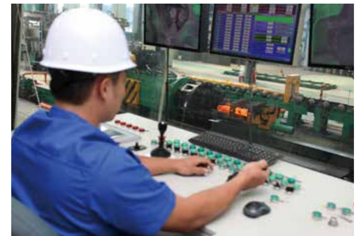
▲ Radial Forging Control Room
